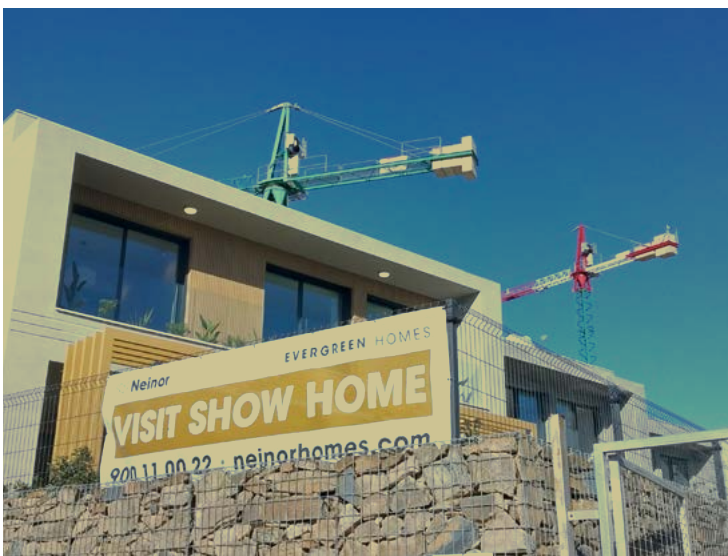
This under-construction site called Evergreen Homes – El Chaparral is at Mijas, a 40-minute drive from Malaga. It will offer 80 townhouses of 3 and 4 bedrooms right next to the El Chaparral golf course. It was acquired from Kronos in 2018 and construction started last year. It is aimed at foreign buyers
